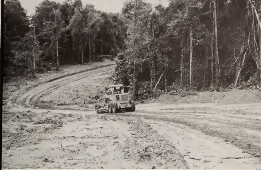
Building a new road through the dense vegetation of the interior Courtesy Leslie B. Johnson, Sr.
